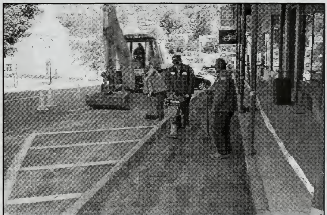
Main Street sidewalk under construction (near the corner of Grove and Main Streets)
