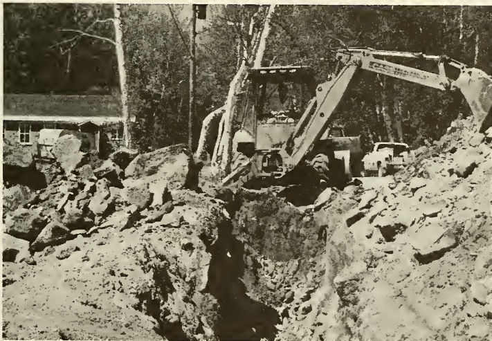
Water and Sewer Department installing 1,300 feet of new 10 inch water main into Perkins Brook Watershed.
