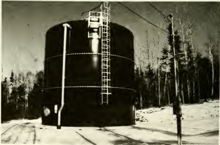
Water Storage Tank at Cherry Mountain
