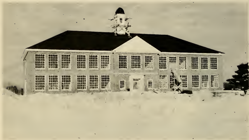
The new Hood Memorial School will house the 7th, 8th, and 9th grades. At the time of this picture the school is about 80% complete. It will be finished in June, ready for classes in September.
