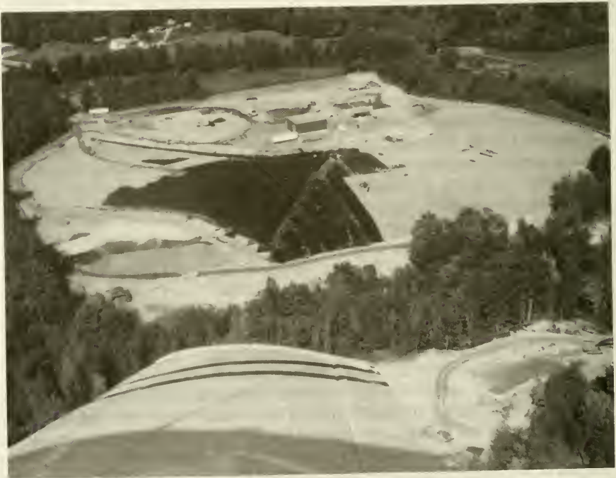
Solid Waste Facility Landfill Closure under construction. Photo courtesy of Eric Meador.
