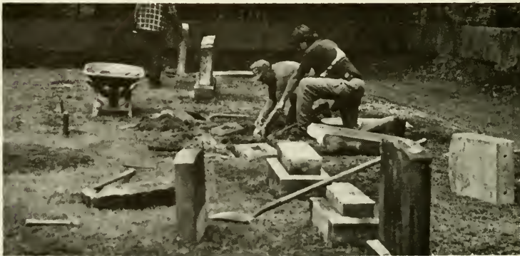
Headstones being repaired in Davidson Cemetery by Public Works Dept. employees - Fall 1990
