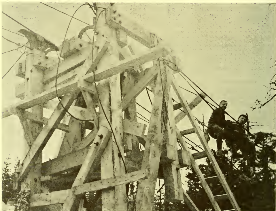
This is the top terminal of the freight tramway. It was located in back of the present Mountain Station. The vertical sheave reversed the pull rope direction from the valley power source to the car.
