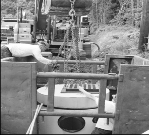
Photograph of the installation of a pre-cast concrete catch basin in preparation for the reconstruction of Stagecoach Road.
