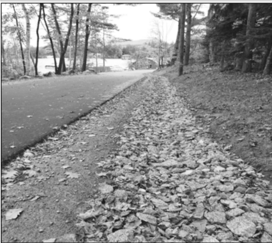
Photograph of Burkehaven Hill Road (south of Lake Avenue) reconstructed between Lake Avenue and Burkehaven Lane.
