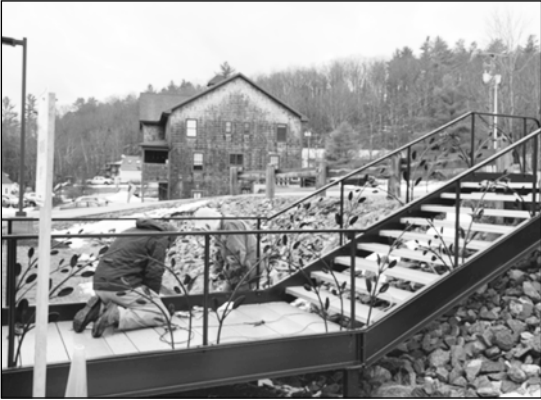
Beautiful new railing by J.A. Metalcraft—thank you to the Foundation for donating this to the library
