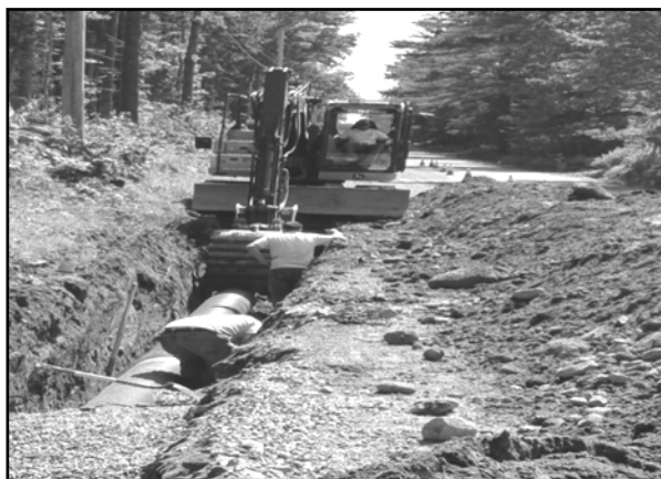
Photograph looking north to south along the east side of Ryder Corner Road of the installation of the 15" HDPE trunk line
