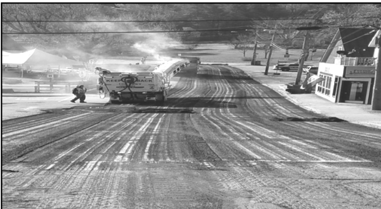
Photograph of Main Street coming into the Harbor being cold planed in preparation for re-surfacing.
