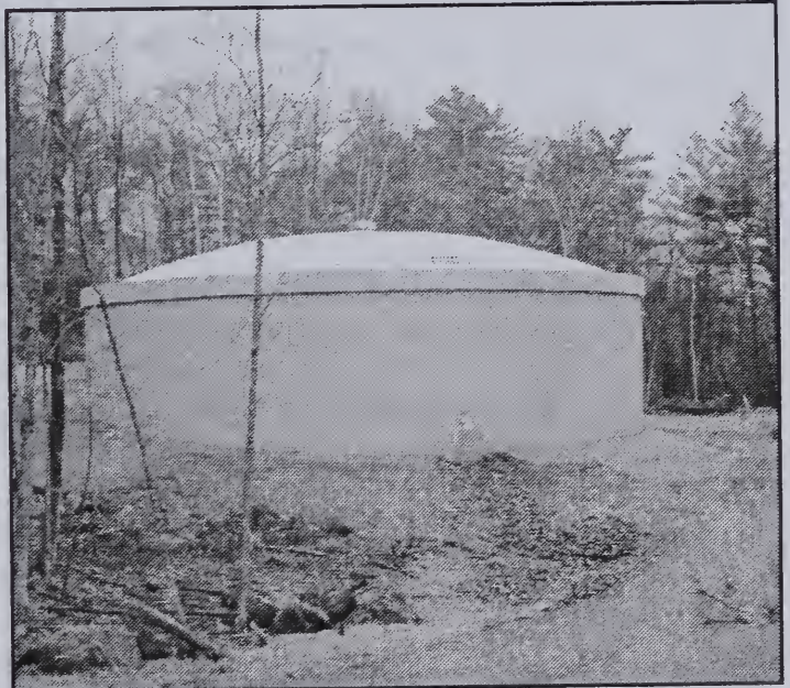
New Water Tank on Route 124
