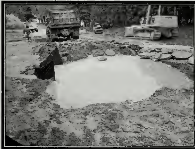
Smith Avenue Washout
