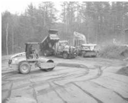
Highway crew member Pat Moore is operating the roller during the site work improvements at the Transfer Station.
