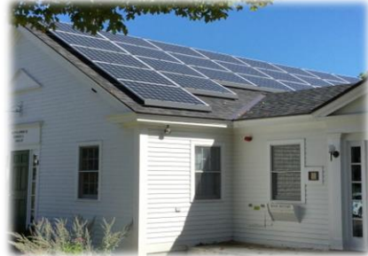
Solar panels on Library Roof 2015
