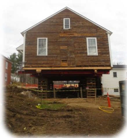
Rear view of Town Hall in fully raised position
