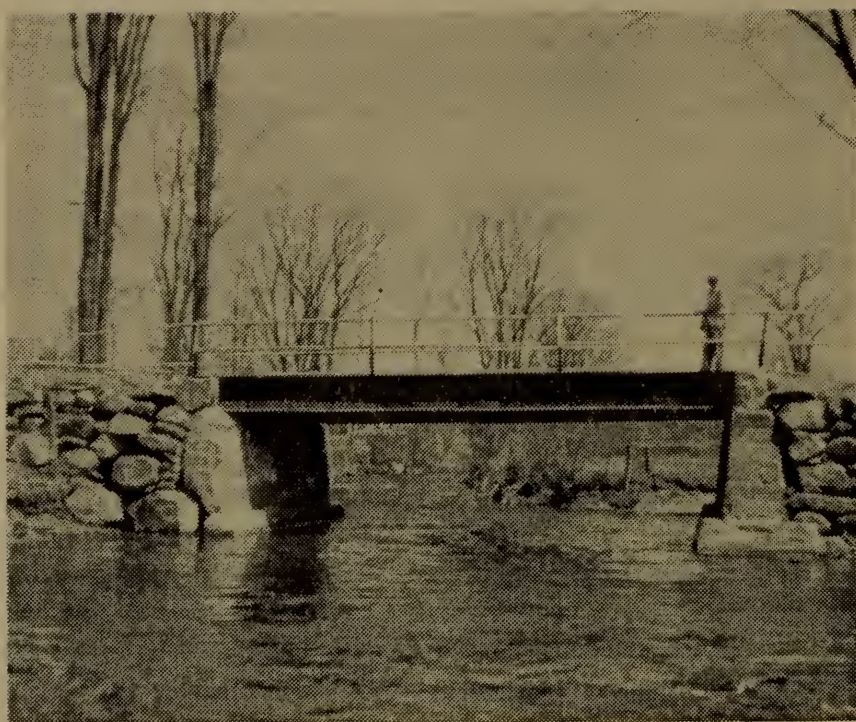
Old bridge on North Road over Garland Brook. It was damaged later by flood.
