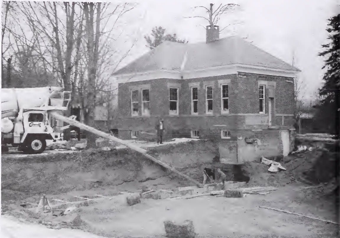
Library expansion: foundation footings being poured as project supervisor David Grobe looks on. —Nancy Norwalk photo
