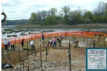
Assess damage and plan for restoration
