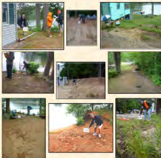
Examples of Identified Erosion Problems
