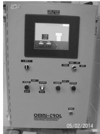
Pump Station Control Panel
