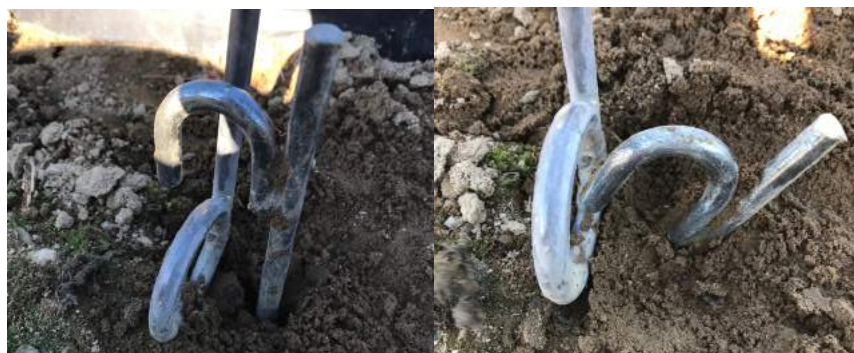
Fig. 31: Grounding stake installed vertically (left) and at an angle (right) onto the peg at the base of the low tunnel hoop. Photo: K. Orde
