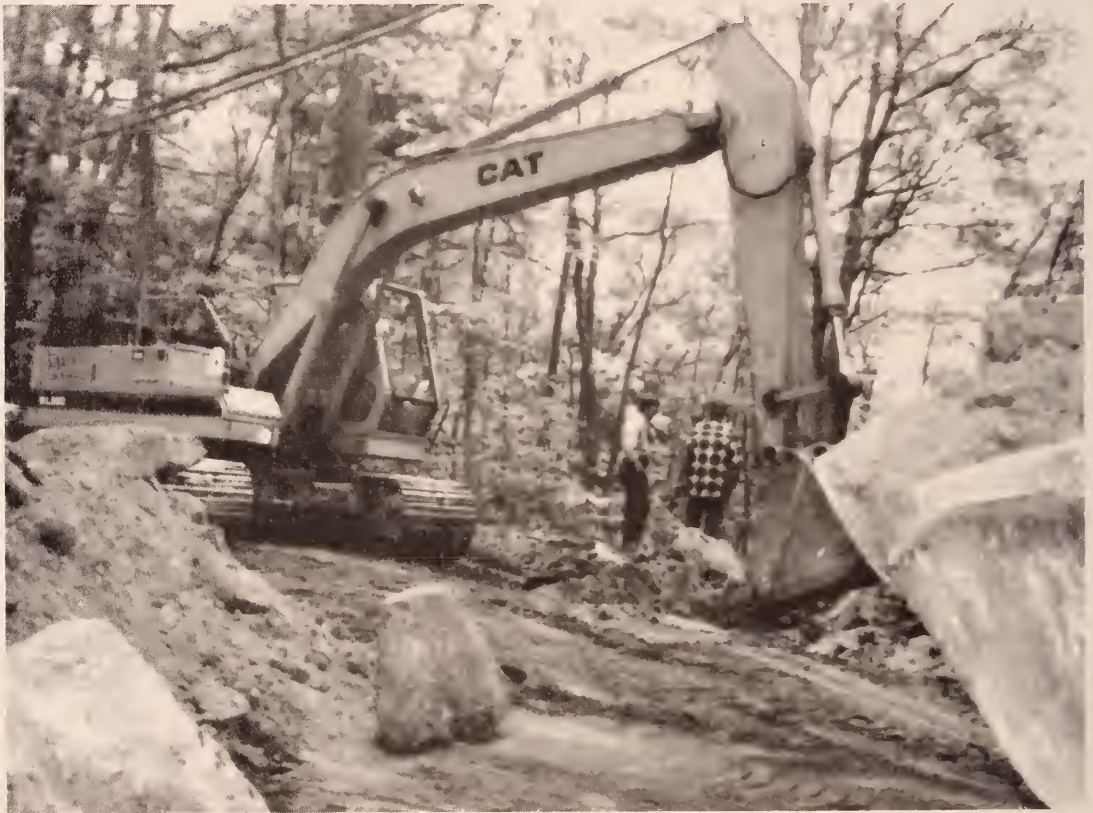
Keyser Street Improvement (Bond): Widening and clearing at top of Pillsbury Hill.
