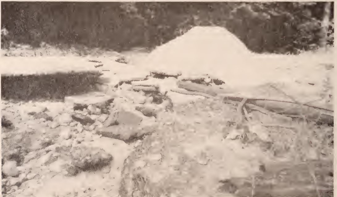
Washout on the Roby Road, August 7, destroying pavement and making the road impassable.
