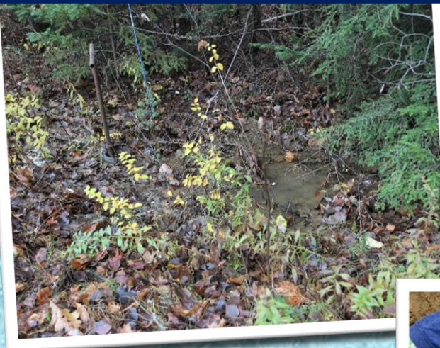
A water break can look like this above ground ...
