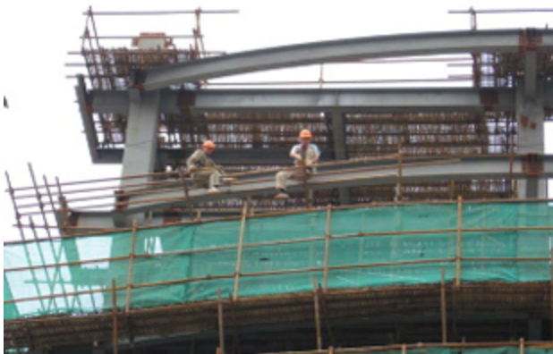
New supported by the old: in Shanghai, bamboo scaffolding is used for construction of modern high-rises (Susannah Pratt.)
