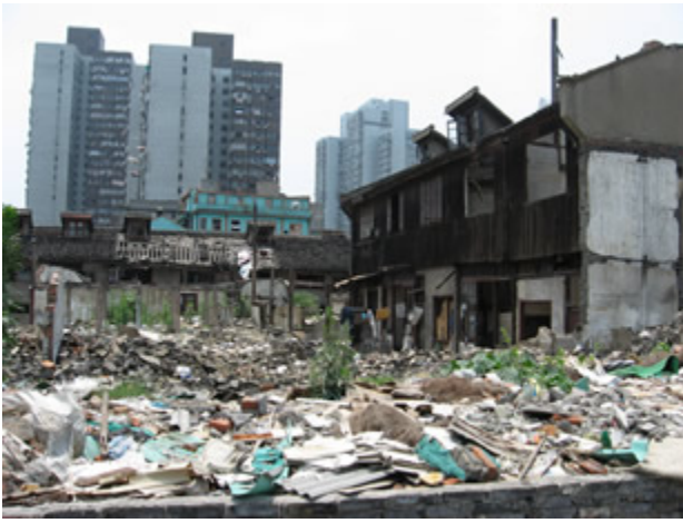
The aftermath of government demolition to a low-income housing area in western Shanghai.
