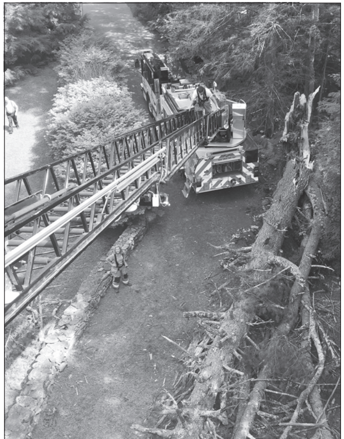
Firefighters use the ladder truck to patch damage to a home located off of Little Sunapee Road, after a large pine tree was taken down by strong winds.
