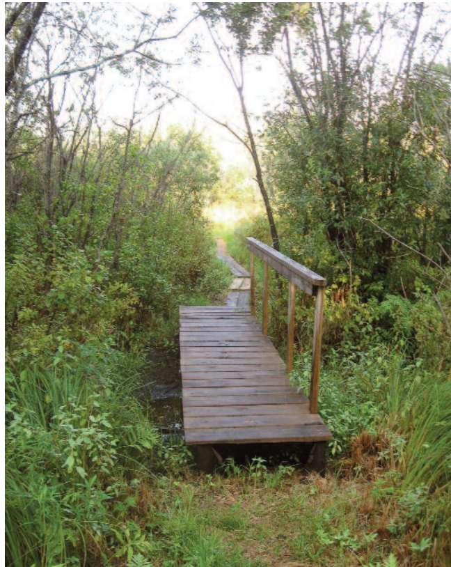
A new bridge installed at the Kidder-Cleveland-Clough Trail. Photo courtesy of Mike Gelcius.
