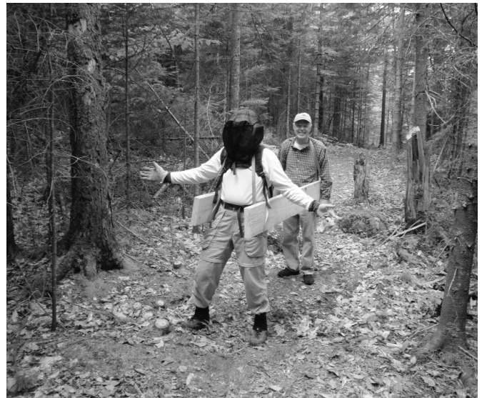
Dan Allen and Bob Lavoie carry bridge construction material into the Lyon Brook trail.
