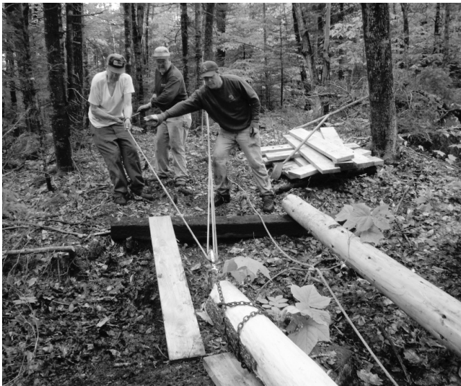
Conservation Commission members Dan Allen, Bob Brown, and volunteer Andy Hager build new bridge on Lyon Brook trail.
