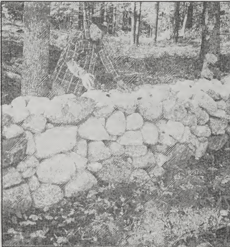
Walter Mains of Ela Mill Road building stone walls at the Town Meeting House. (Photo by Eloise Bickford)
