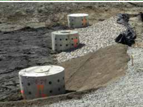
Subsurface gravel wetlands have demonstrated exceptional water quality treatment in a range of land uses, including commuter parking, high-density commercial development, and along major transportation corridors.
