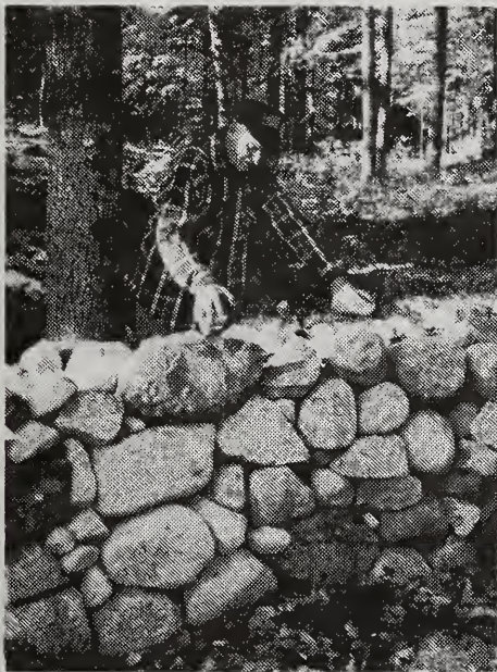
Walter Mains of Ela Mill Road building stone walls at the Town Meeting House. (Photo by Eloise Bickford)
