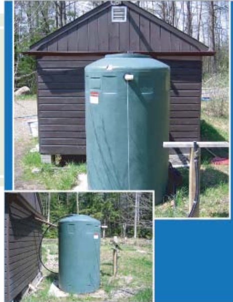
550 gallon cistern installation collecting rainfall runoff from a guttered roof.
