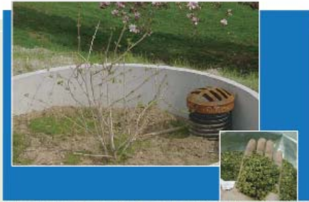
Bottomless tree box filter after installation (left). Close-up of the coarse sand-compost media used in the tree box filter. The 76% coarse sand/24% compost mixture has 10% organic matter and infiltrates water at a rate of 14.6 inches/hour in the laboratory (right).
