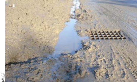
Construction site erosion near storm drain
