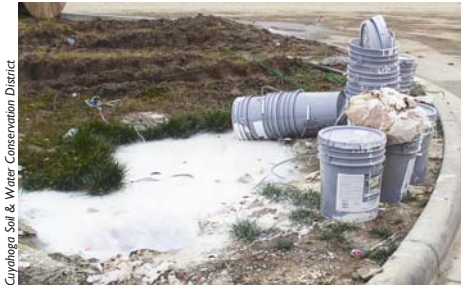
Paint spill at construction site
