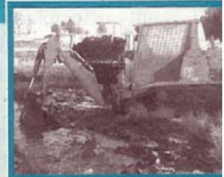
The specialized low ground pressure excavator and dump carrier used to implement this restoration work exerts about two-pounds/square inch of pressure on the surface of the marsh (less than a human footprint).
