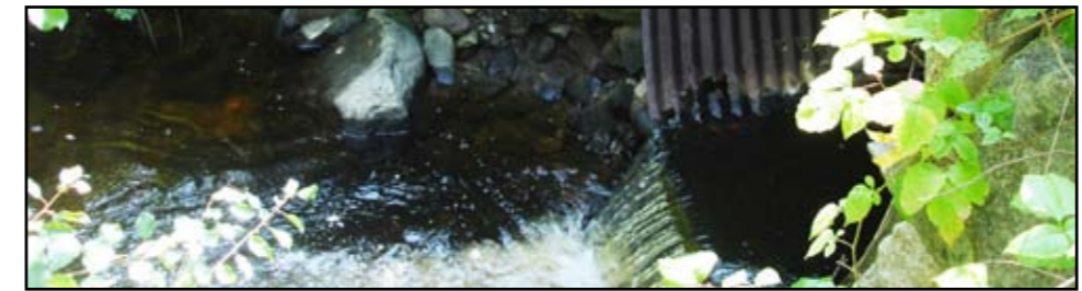
Culvert on Thompson Brook in Greenland is a barrier for some migratory fish.
