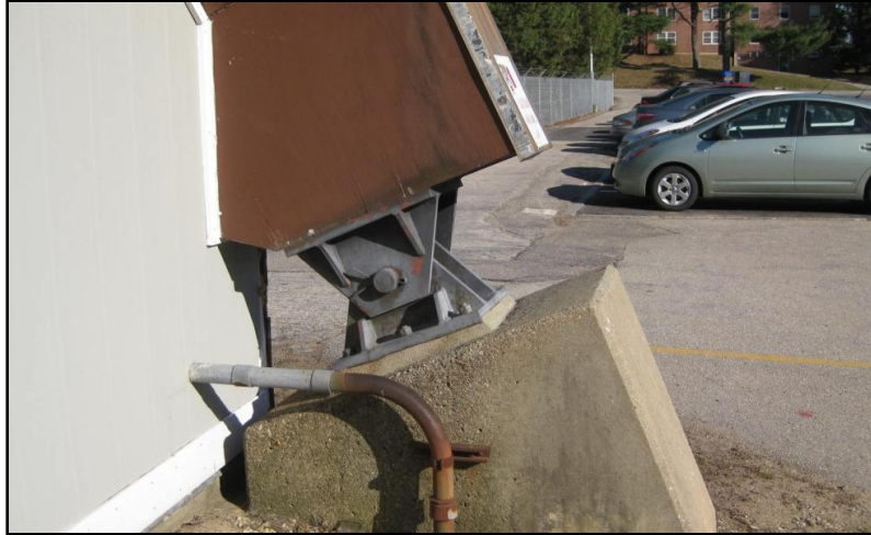
Figure 5: Steel hinge at the end of an arch at UNH's Wittmore Center
