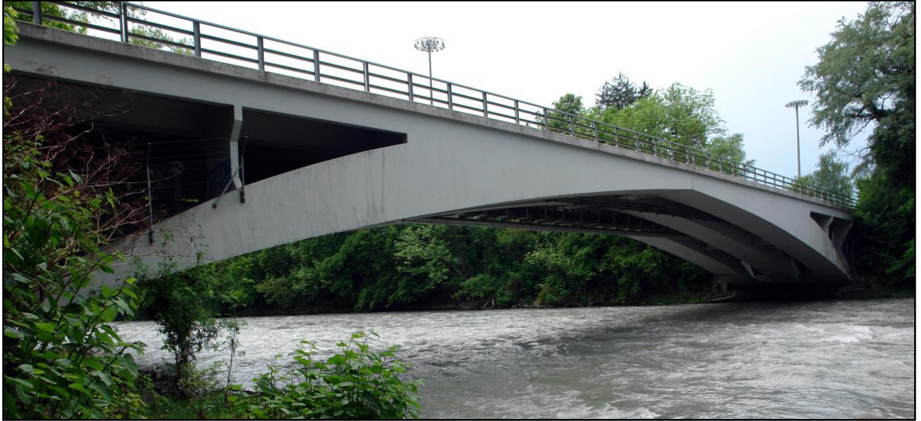
Figure 32: Maillart's bridge at Vessy - note the variation in rib depth (Wikimedia Commons)
